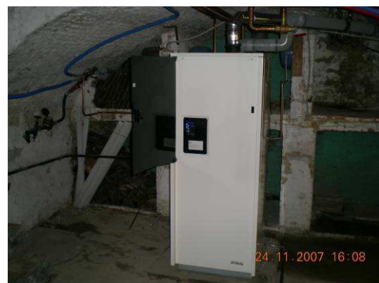
Figure 1.7: nouvelle chaudière → NO x = 1,5 kg/an
