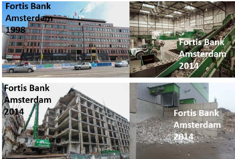
Figure 7: representative example in Amsterdam where the building is demolished earlier than expected. (Durmisevic et al., 2016)
