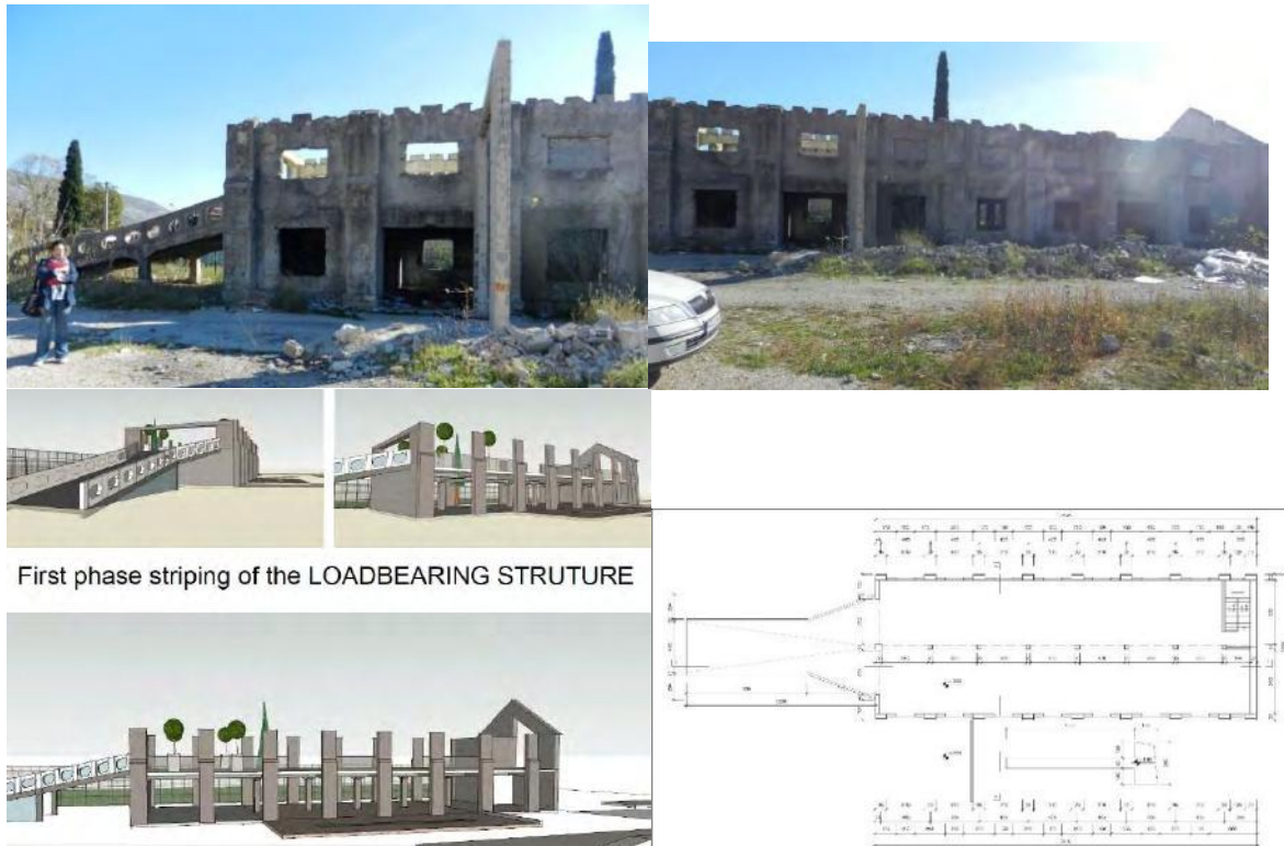
Figure 15: Representation of the existing building structure and the image of the building after removing all infill elements (non-structural elements).
