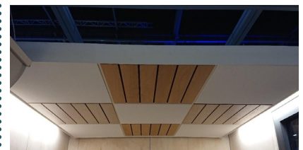
Figure 55: The Armstrong ceiling combined with the wooden NON ignis ceiling panels was installed in the office unit from Ecobuild onwards. The canopy construction also allows for side lighting.
