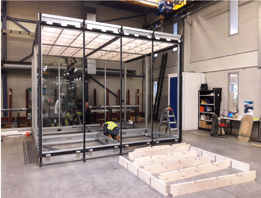
Reversible wooden roof cassettes were assembled within the metal frame of the GTB lab module. They were produced by the Delft based start-up: The NewMakers.
